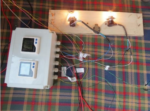
Figure 3. DC Energy meters connected to load
