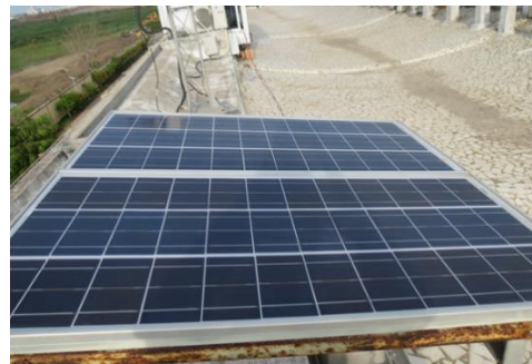
Figure 1. 80 W Solar Panels
