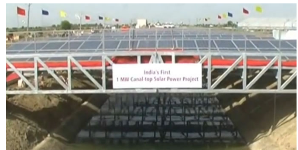
Figure 2, Glimpse of India's first Canal Top Solar PV Plant installed in Gujarat.
