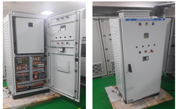
Figure 1: Interior and exterior view of the 20 kVA hybrid inverter
